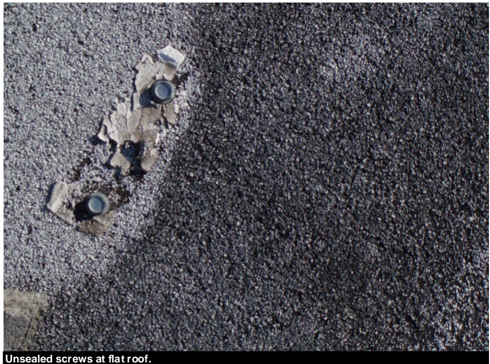
Unsealed screws at flat roof.
