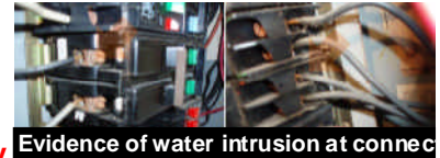
Evidence of water intrusion at connec
