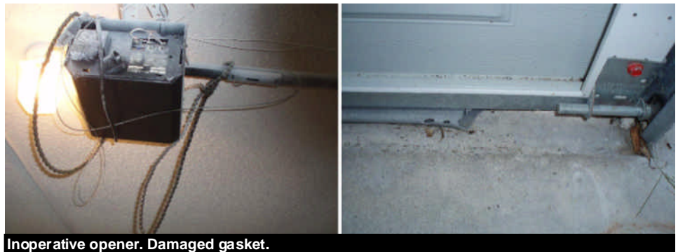
Inoperative opener. Damaged gasket.
