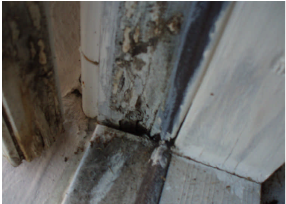
Deterioration garage service door.
