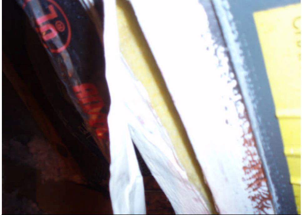
Return air leak at air handler. Tape loose
